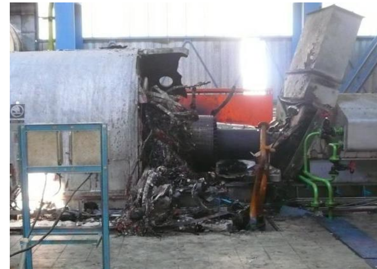
Iranshahr Thermal Power Plant rotor angle instability event 2009 [4]
