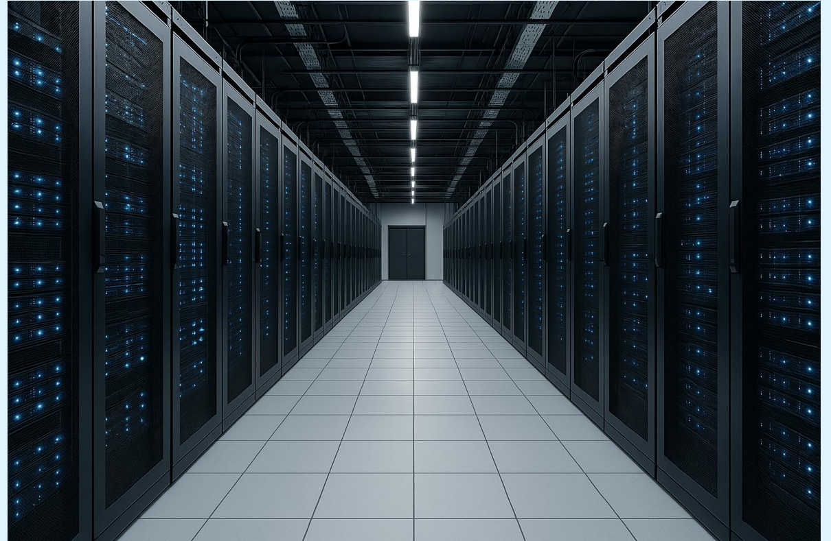
Example data centre interior
