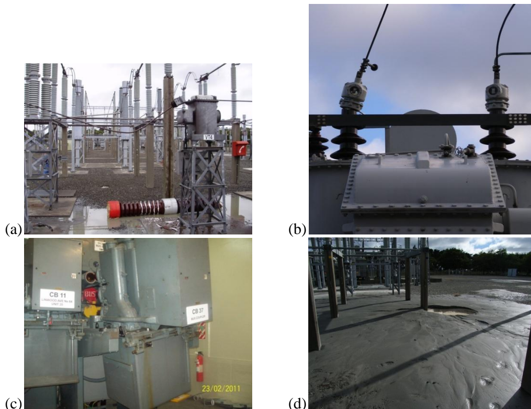
Figure 6: Bromley Substation (Photos: Transpower)
