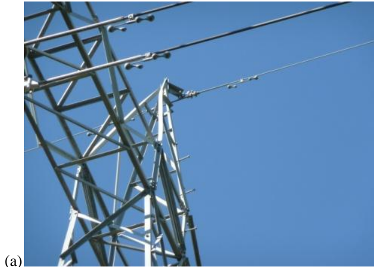
Figure 9: Benmore-Islington A line (Photos: Transpower) (a) Earth peak bent on tower 600.
