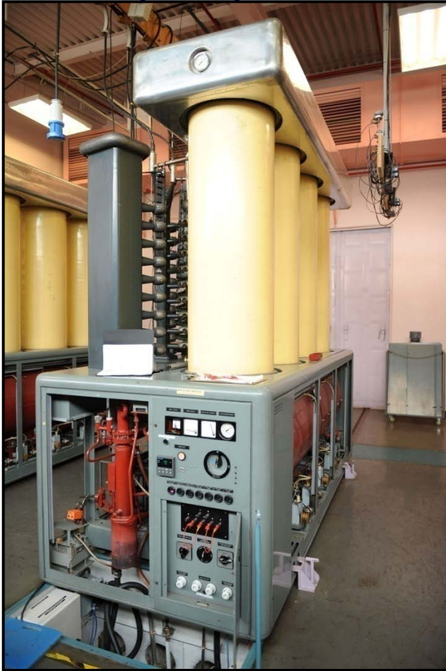
Pole 1 – Mercury Arc Valves (1965)
