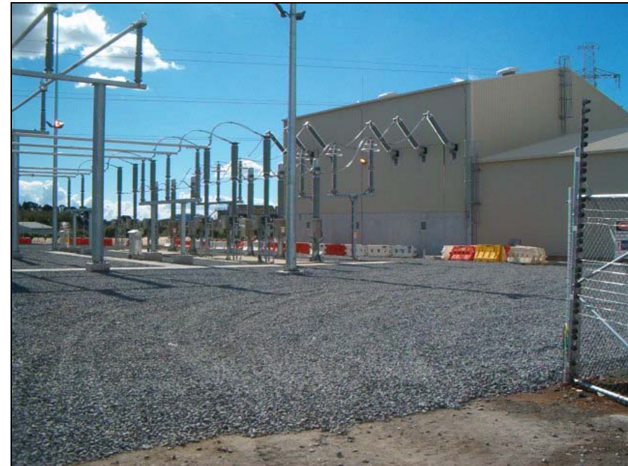
AIS switchyard with connection to GIS building and switchgear – April 2010
