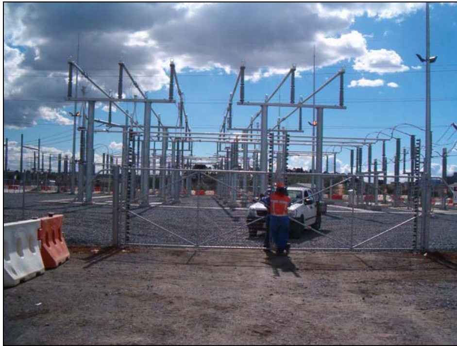
New AIS switchyard – April 2010
