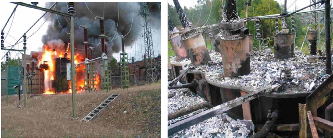
Figure 3: HVDC Converter Transformer Fire (Konti-Skan 1, Sweden)
