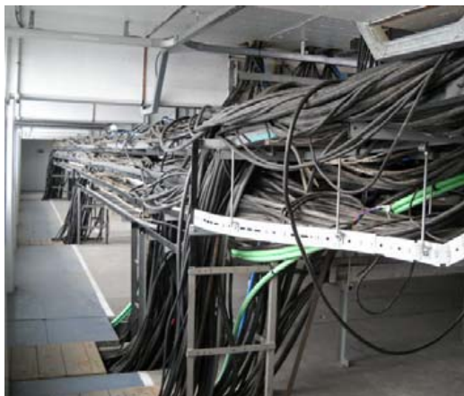
ISL cable basement – general view
