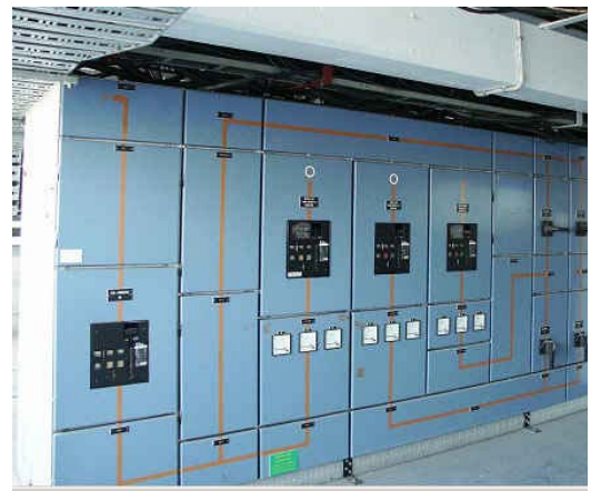
Main 415 V LVAC switchboard
