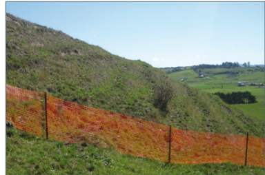
Fencing erected to visually demarcate a Pa site to be protected during transmission line construction activities.
