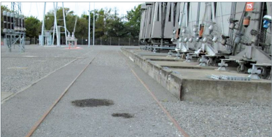
Oil stain from historic contamination associated with a former transformer bund discharge.
