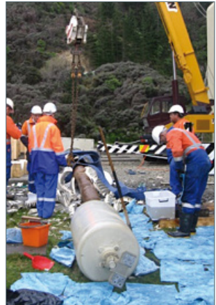
Clean up of oil resulting from a dropped bushing.
