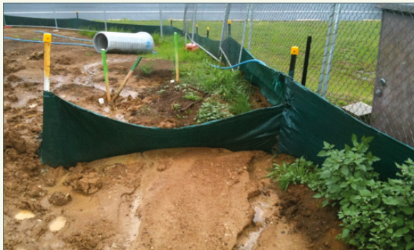
This sediment control fence return badly needs maintenance to prevent the sediment bulk over whelming the fence.
