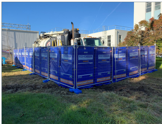
Echo noise barriers deployed around truck undertaking hydrovac excavation near residential properties.
