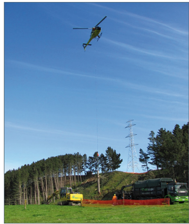
Helicopters were used on the construction of the NIGUP transmission line to protect and preserve archaeological sites by minimising both machinery on site and earthworks for access and construction.
