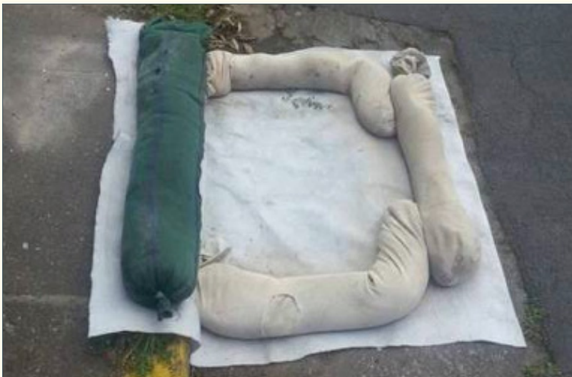
Geotextile sausage and material used to protect a kerb drain. A geotextile sump bag would be better still but must be regularly inspected and emptied.
