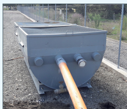
Baffle tank and discharge pipe.
