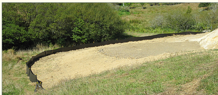
Sediment control fence installed along the contour to control sediment runoff from a large area of earthworks.
