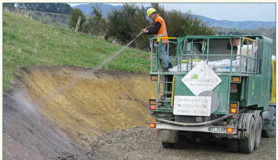
Hydroseeding can provide stabilisation of exposed soil and slope faces by providing for rapid grass growth.
