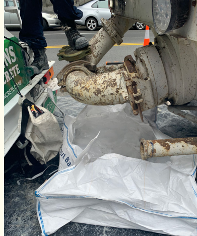
Concrete washout bag in use, tethered to vehicle to keep bag open to receive washout material.
