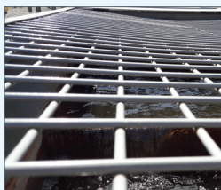
Baffle tank weirs to provide sediment settlement prior to discharge.
