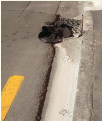
Poor implementation and maintenance of controls can lead to concrete discharge.
