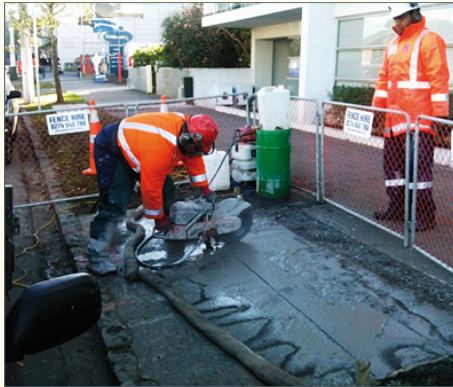
A nice example of potential controls during concrete cutting including placement of a barrier to water discharge.
