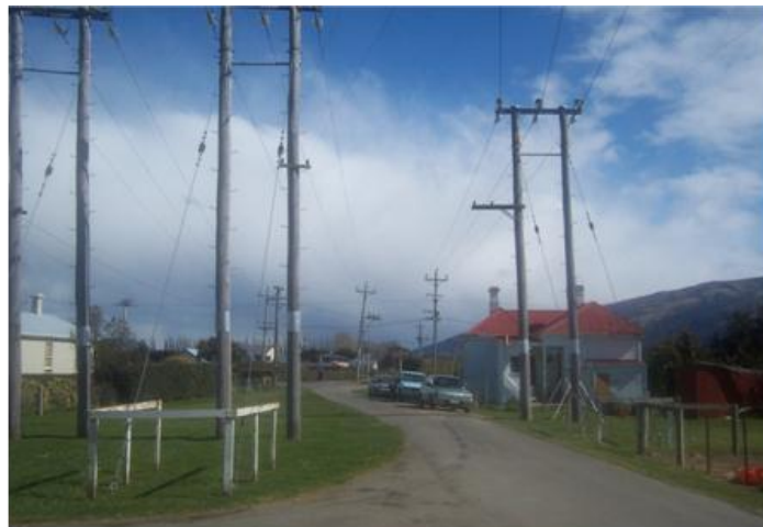
Figure 11 - 33 kV Subtransmission Lines at Outram
